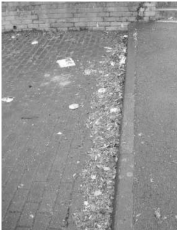
Litter and detritus accumulation in car parking bay, built up over time
