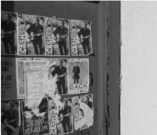
Fly-posting on disused building doorway
