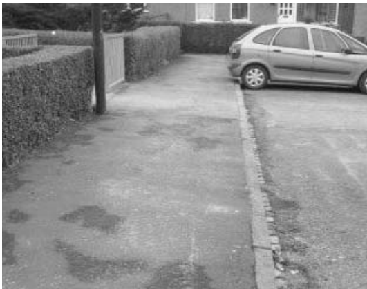
Significant weed growth in the channel
