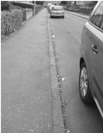
Litter and detritus accumulating in the channel, cars routinely parked by kerbside.
