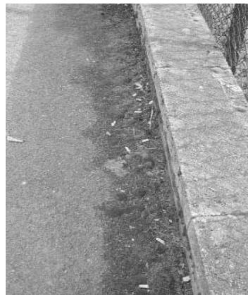
Significant weed growth along backline as well as cigarette ends
