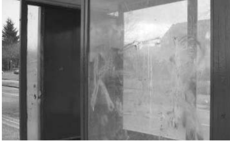
Graffiti on bus shelter, panels vandalised (etched writing)
