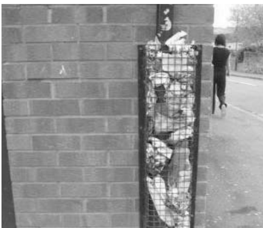
Litter forced into building vent guard, collected over a prolonged period
