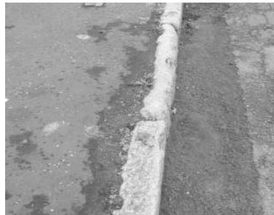
Weed growth impacting along gaps appearing between kerbstones and pavement
